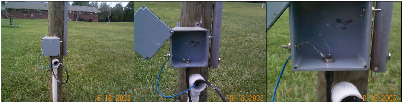
The box at the bottom (with resistors and small inductors) resonates the vertical to 1830 and brings the R value up to 75 ohms. The feed line goes to a center matching, switching, delaying unit.
